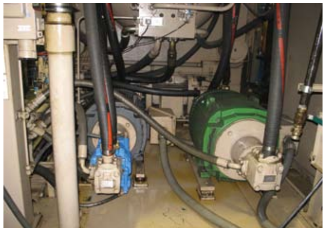
Cryogenically-treated hydraulic pumps installed on a machine at Rantoul Products.
