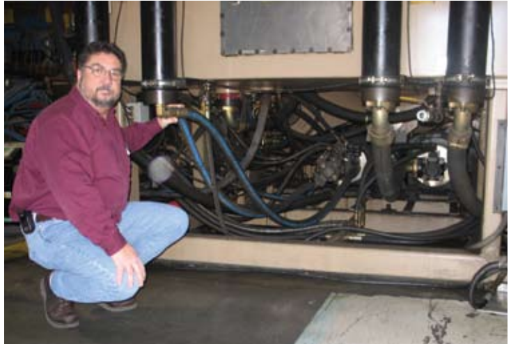
Waller inspects these cryogenically-treated hydraulic pumps installed on a machine.
